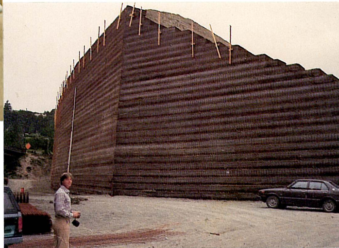
← SEATTLE PRELOAD Welded Wire Retaining Wall, 18" Lifts Seattle, Washington Washington Department of Transportation Contractor: E.L. Grice and Sons
