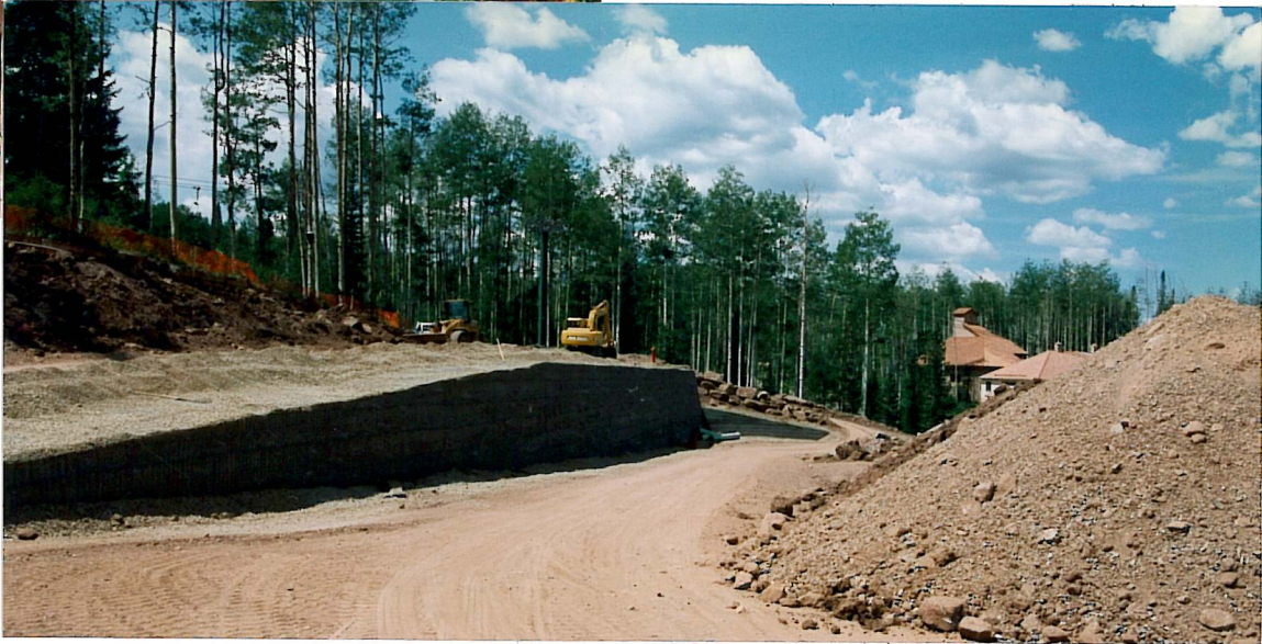
TELLURIDE PARKING STRUCTURE Welded Wire Retaining Wall, 24" Lift (11,856 Sq. Ft.) Telluride Mountain Village Owner: Metropolitan District Contractor, Shaw Construction Designed By: MacIntosh Engineering and Development. October/November 1995
