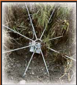
Left, Spiralnail attached to a Spider. This Spiralnail is one of 50 Spiralnails, including Spiralnail drains, used to complete a slide repair project along North Camano Drive in Washington. The Spiders attached to the Spiralnails reinforce and confine the face of slope through existing vegetation and around existing trees. Presently, this is the only method available for repairing or stabilizing steep slopes that leaves the existing vegetation and trees intact.
