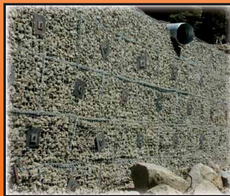
On Left is a finished Gabion Faced Spiralnail Wall located in Humboldt County, California. This wall was constructed using the method described above.
