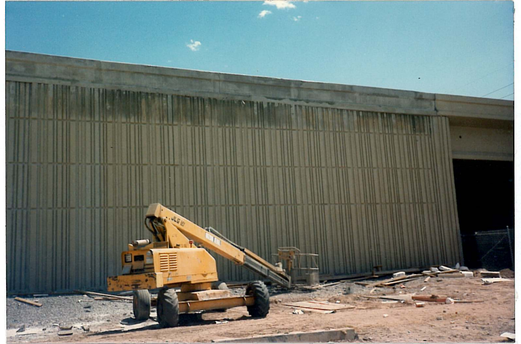
EHRENBERG-PHOENIX HWY. (I-10), Phoenix, Arizona Arizona Department of Transportation Contractor: JWW Contracting Co., Inc. Summer - Fall 1985
