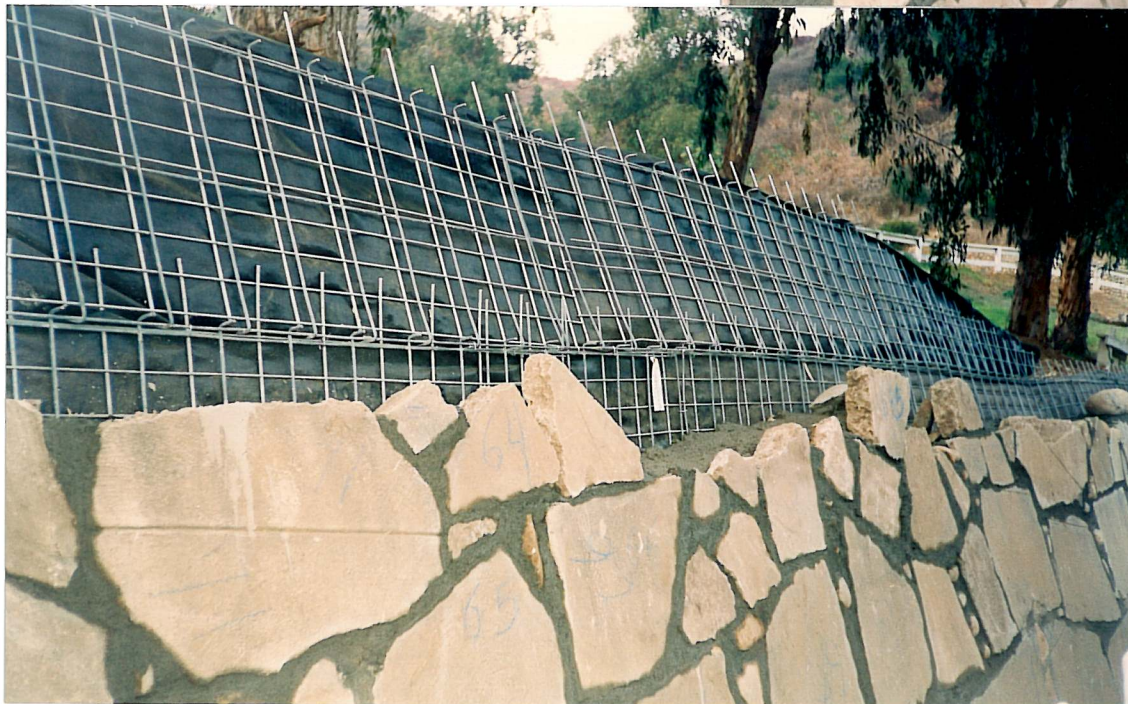
WILL ROGERS STATE HISTORIC PARK Welded Wire Retaining Wall, 24" lift (1856 Sq. Ft.), Rock-Faced Los Angeles County, CA State of Calif. Dept. of Parks and Recreation Contractor, J&A Development Designed By: Dept. of Parks and Recreation October 1994
