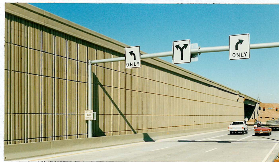
Eureka Reinforced Soil (Cast-in-Place Face) ARIZONA DEPARTMENT OF TRANSPORTATION EHRENBERG ROAD Phoenix, AZ JWJ/Valley
