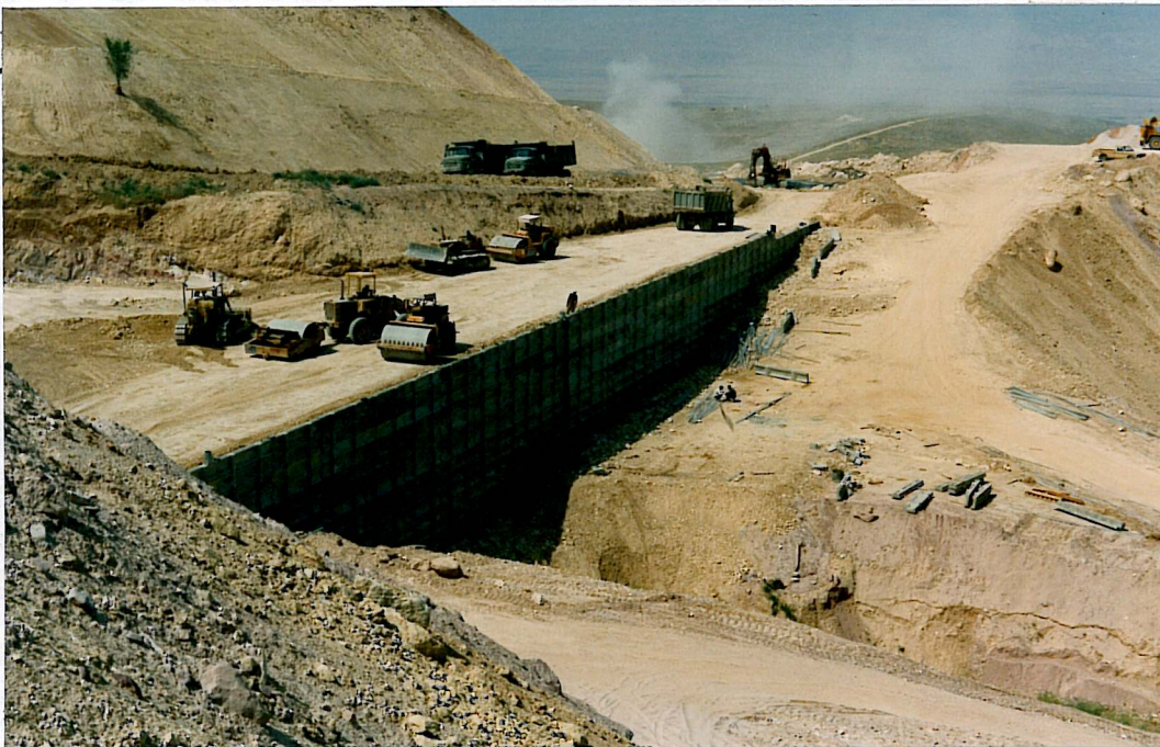
Reinforced Soil Embankment-Shadow Panel Dead Sea Highway, Amman, Jordan Jordanian Ministry of Public Works, Summer 1990
