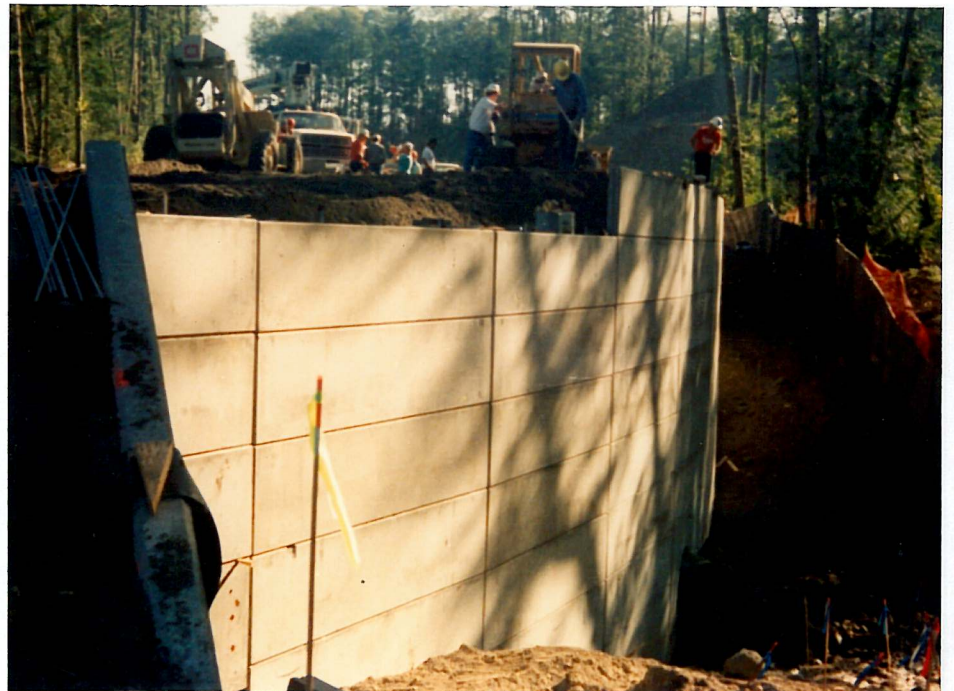
HARBOUR POINTE INDUSTRIAL PARK RSE - Smooth-Face Retaining Wall Mukilteo, Washington Contractor: Tri-State Construction & Roger G. Young, Inc. Fall 1991 41,372 Sq. Ft.,
