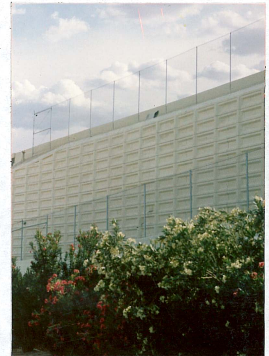
Reinforced Soil Embankment (Shadow Panel) NEVADA DEPARTMENT OF TRANSPORTATION/U.S. 395 Las Vegas, NV Contractor: Riggs/Valley
